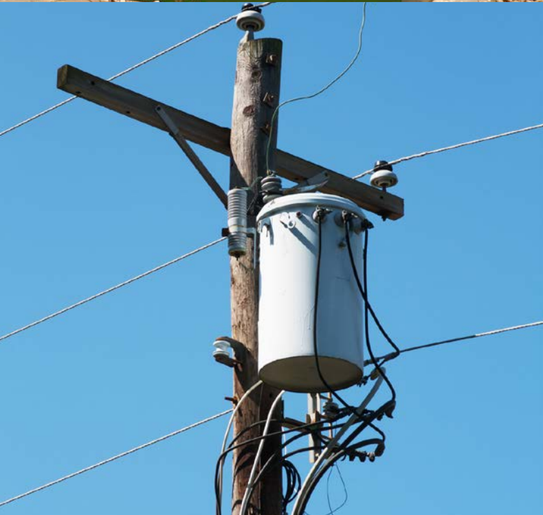
While pole-mount transformers account for the most orders of transformers by numbers [23], pad-mount demand is expected to increase as utility investment in undergrounding and resilience programs increases. Photos from Getty Images, top: 1388647482, bottom: 152264156
